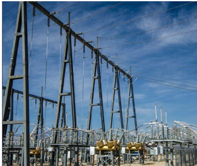
Transmission Facility In Coachella Valley
