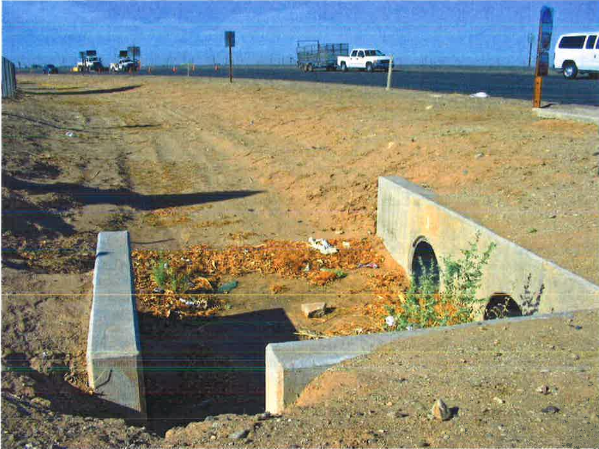
Existing drainage facility at the southwest corner of State Route 7 and Menvielle Rd, facing southwest
