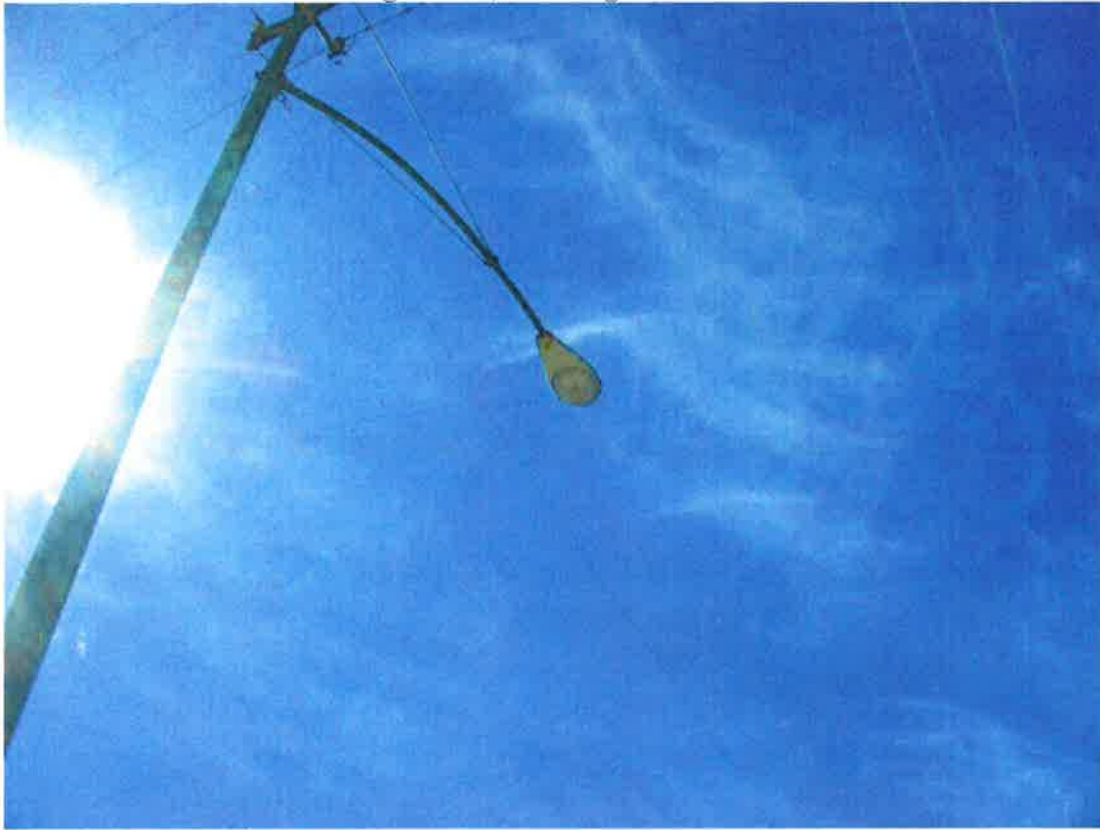
Existing streetlight located on Highway 111
